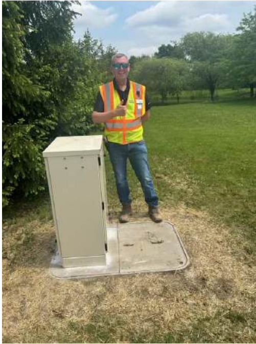
Fiber Distribution Hub (FDH) Approximately 90 to throughout the City
