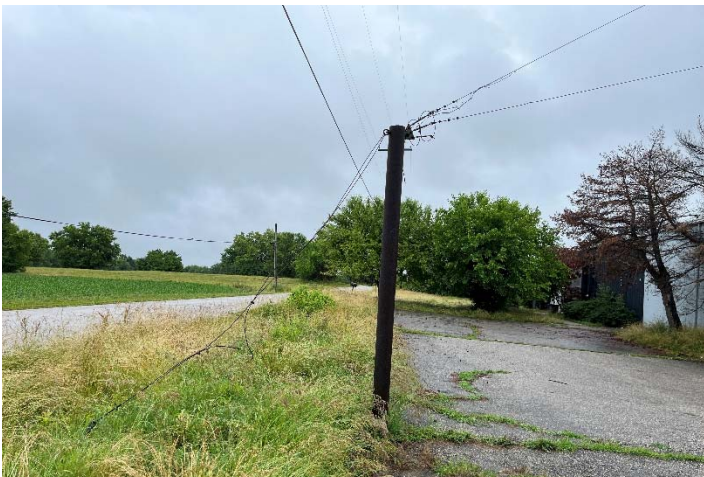
Figure 5. Telecommunication Tower Support (1 of 3)
