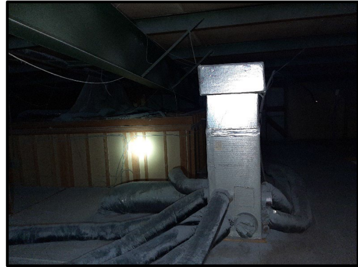
22 – View of ducts with fiberglass insulation above offices
