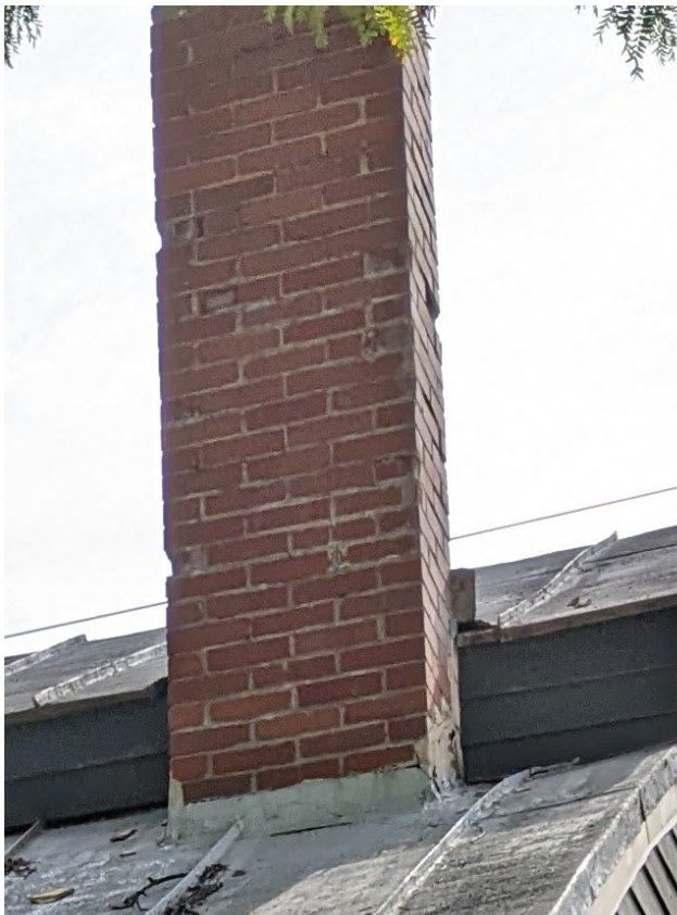
BRICK ON THE NEW CHIM- NEY WILL MATCH THIS BRICK AS CLOSELY AS POS- SIBLE (SOUTH CHIMNEY)
