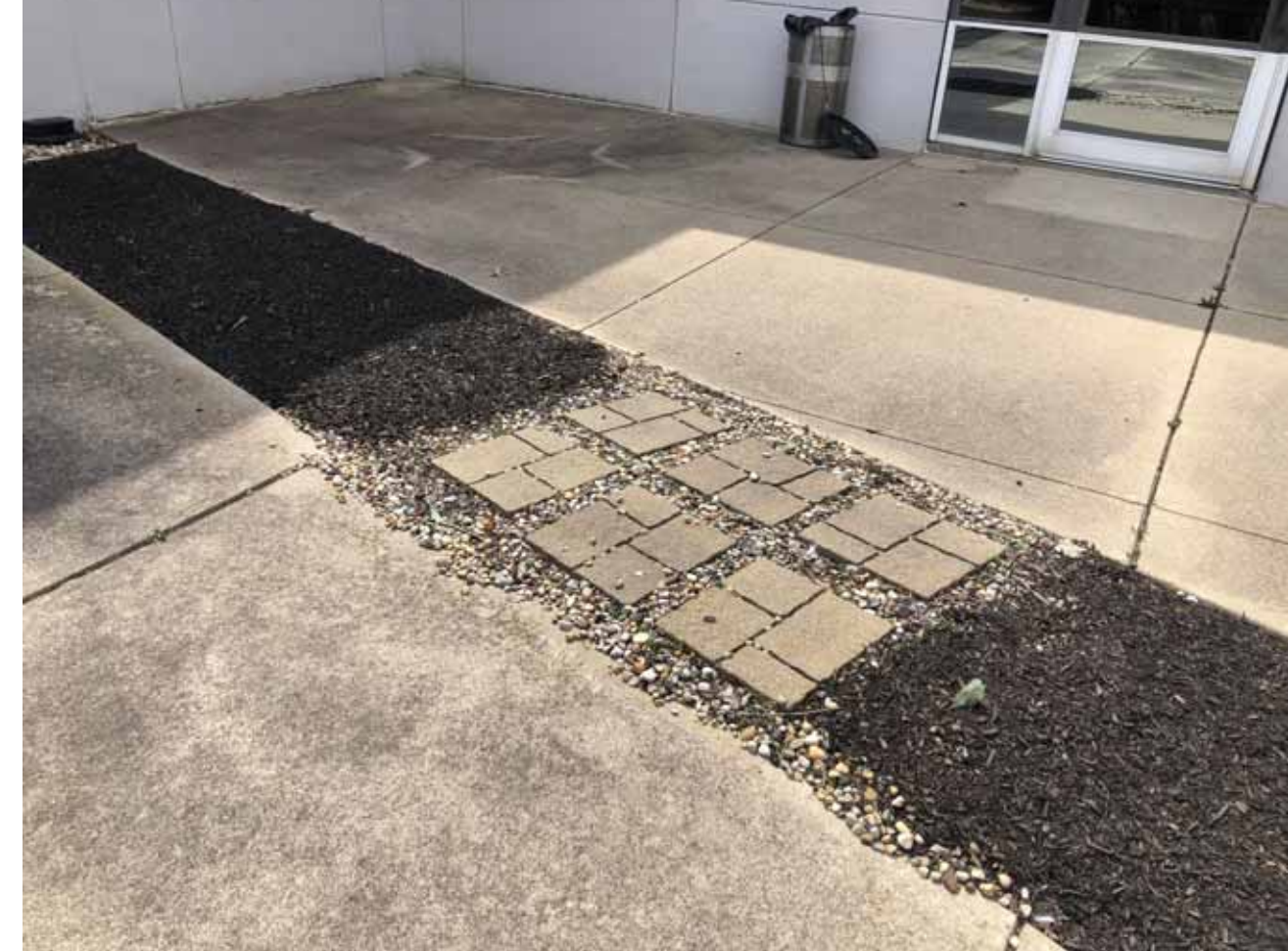
EXISTING SITE PHOTO SHOWING SIX (6) CONCRETE UNIT PAVERS TO BE REUSED IN SAME LOCATION AND RELAYED IN SAME PATTERN LAYOUT DURING CONSTRUCTION. PRESERVE AND PROTECT DURING DEMOLITION. REMOVE WASHED RIVER ROCK AGGREGATE BETWEEN PAVERS AND PAVER BASE COMPLETE.
