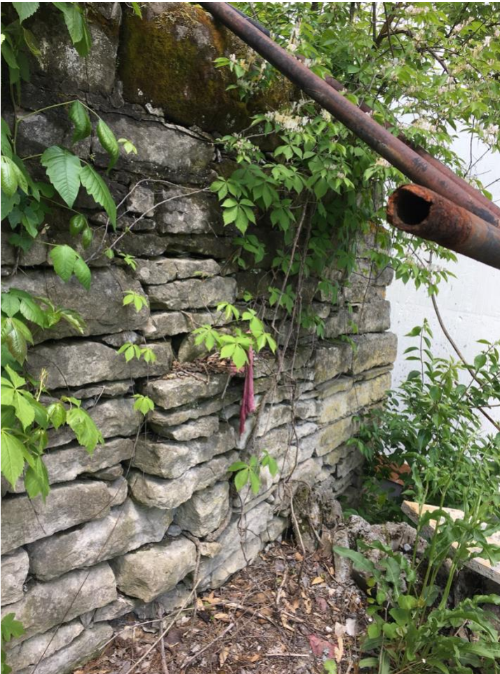
PHOTO 4: Observed concern a few feet south of the northwest corner of the wall where stone appears to be shifting out, bowing similarly to the east wall immediately north of the southeast corner (Preservation Designs, May 2021).
