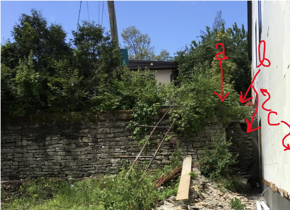
PHOTO 5: Photo of northeast corner (a) of the retaining wall, looking west. From this northeast corner, the wall jogged about twenty some-odd feet west and then turned north. At the time this photo was taken, the retaining wall return was broken (b) just short of then under-construction COhatch building (c) at 25 North Street (Preservation Designs, May 2021).
