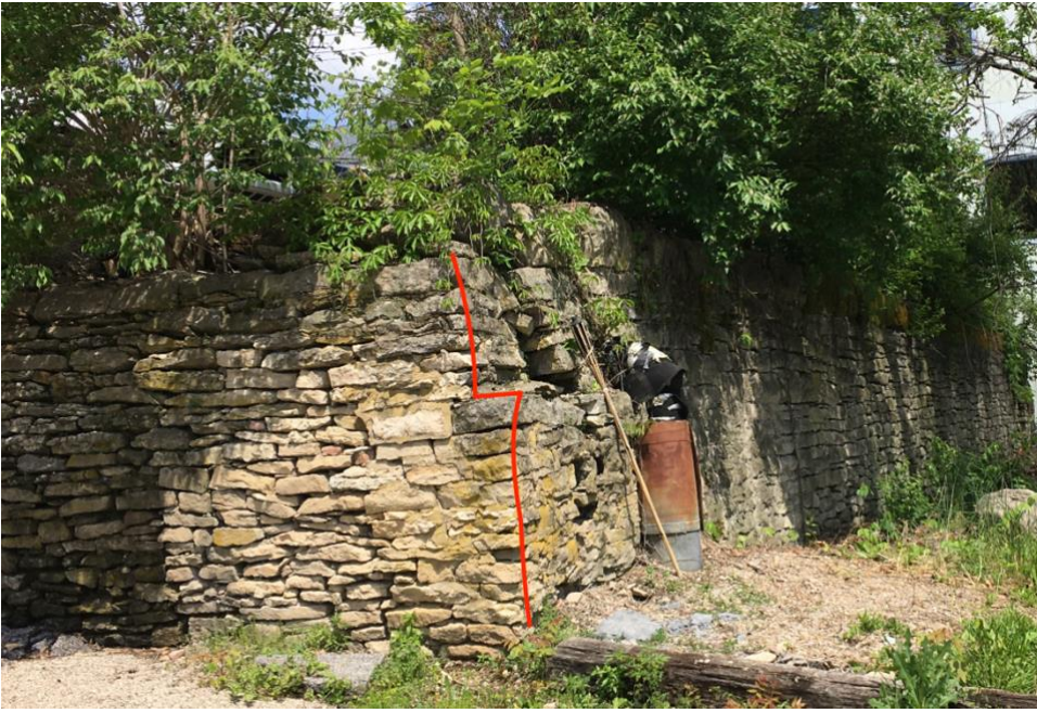
PHOTO 3: Photo of southeast corner of the retaining wall, with a red line highlighting the eastern shift of the lower portion of that wall (Preservation Designs, May 2021).
