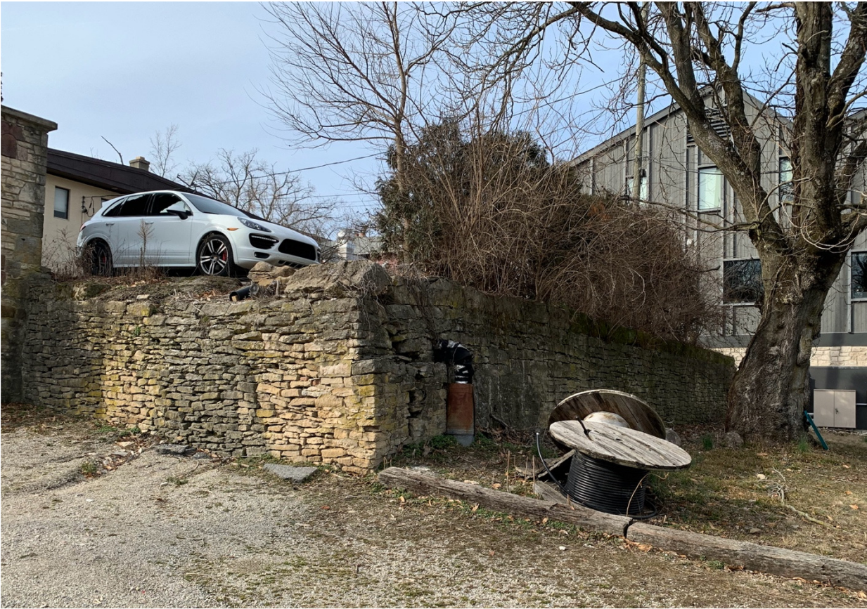
Figure 1. Photograph of the dry-stone retaining wall taken from 38 N High's rear lot looking north-northwest. The bowing wall can be seen in line with the auto's front wheel, as can the lower stones shifted east just north of the southeast corner. The sewer pipe and dry wall joints infilled with mortar lie to its immediate north. (Preservation Designs, February 8, 2023).
