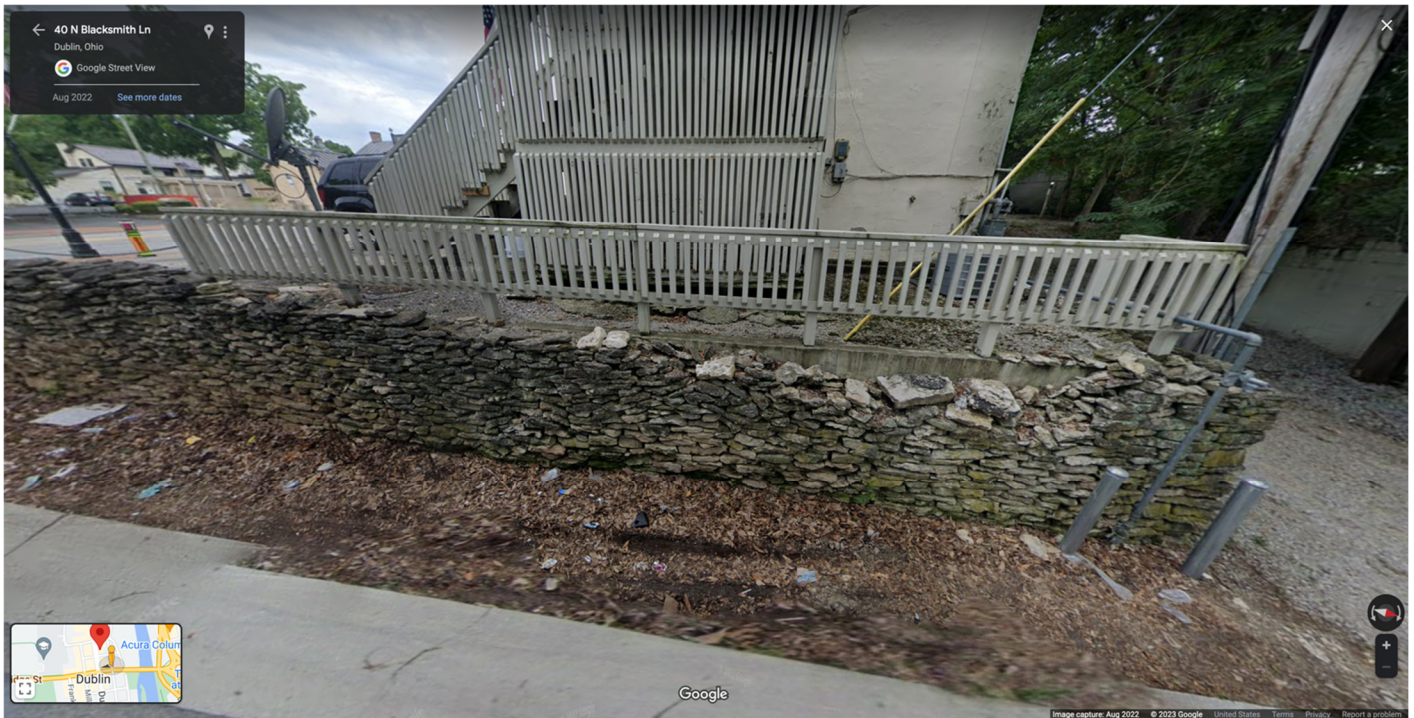
Figure 2. Photograph of a concrete retaining wall with dry stone facing, taken at the northwest corner of N Blacksmith Lane’s intersection with E Bridge Street, looking west. This retaining wall best represents the outcome if Option 2 were chosen; having a single wythe of dry stone loosely stacked against the concrete would need better detailing (including structural ties) to prevent failure and physical loss (Google Maps Street View, August 2022, downloaded February 25, 2023).
