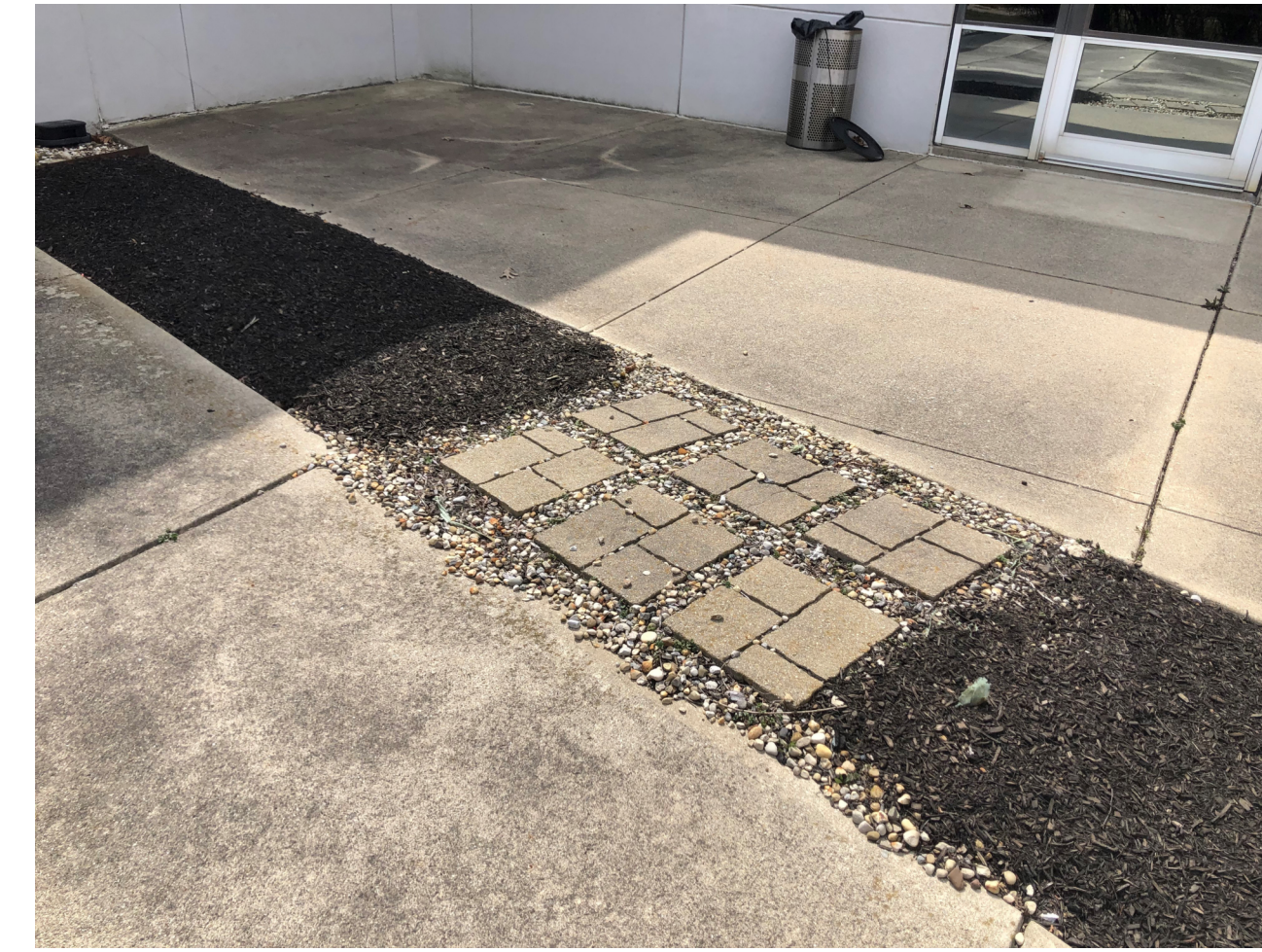
EXISTING SITE PHOTO SHOWING SIX (6) CONCRETE UNIT PAVERS TO BE REUSED IN SAME LOCATION AND RELAYED IN SAME PATTERN LAYOUT DURING CONSTRUCTION. PRESERVE AND PROTECT DURING DEMOLITION. REMOVE WASHED RIVER ROCK AGGREGATE BETWEEN PAVERS AND PAVEMENT COMPLETE.
