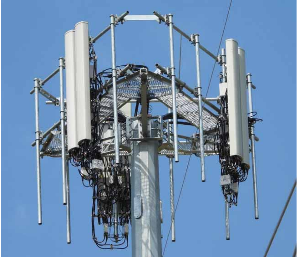
Photo 2: 12 ft. Triangular Platform with Verizon PCS Antennas
