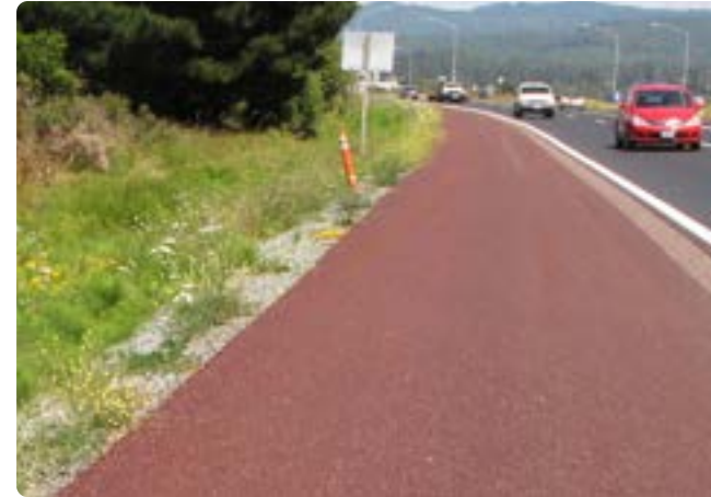
Asphalt paving for trail surface in the Park + Nature Preserve, Suburban + New Development areas
