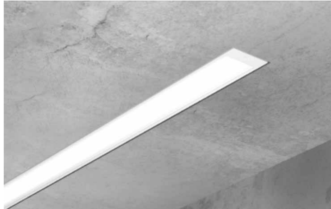
RECESSED LED LIGHT FIXTURE AT ENTRY CANOPIES (USED IN RESI A, B, & C)
