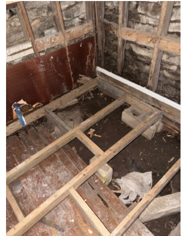
Water infiltration/improvised floor support
