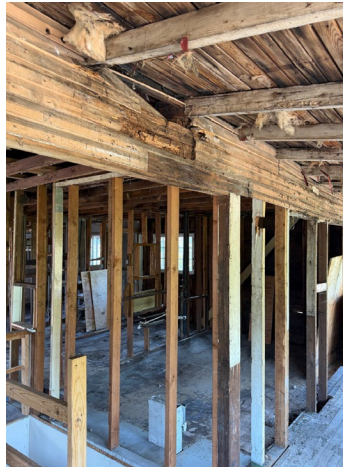
Rotted and sagging beam
