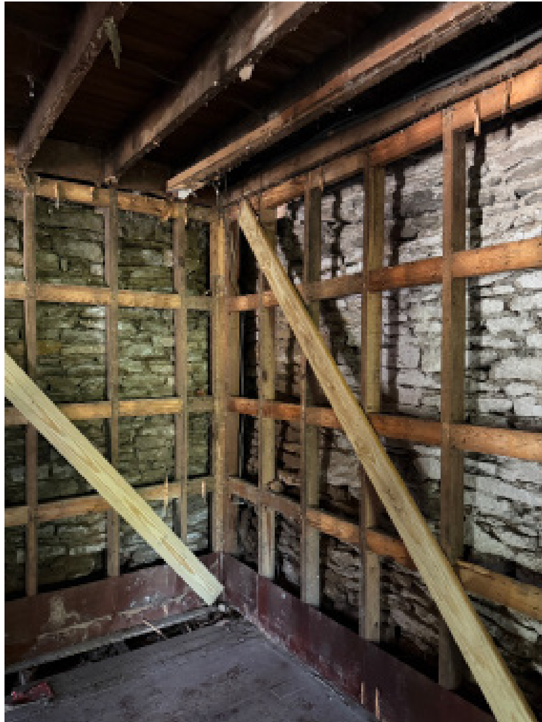
Extensive rotting at the bottom of wall framing against stack stone foundation wall, with groundwater coming in through the gap.
