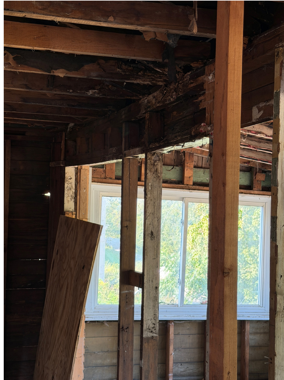
Header wall and ceiling joists are seriously rotted and sagging.
