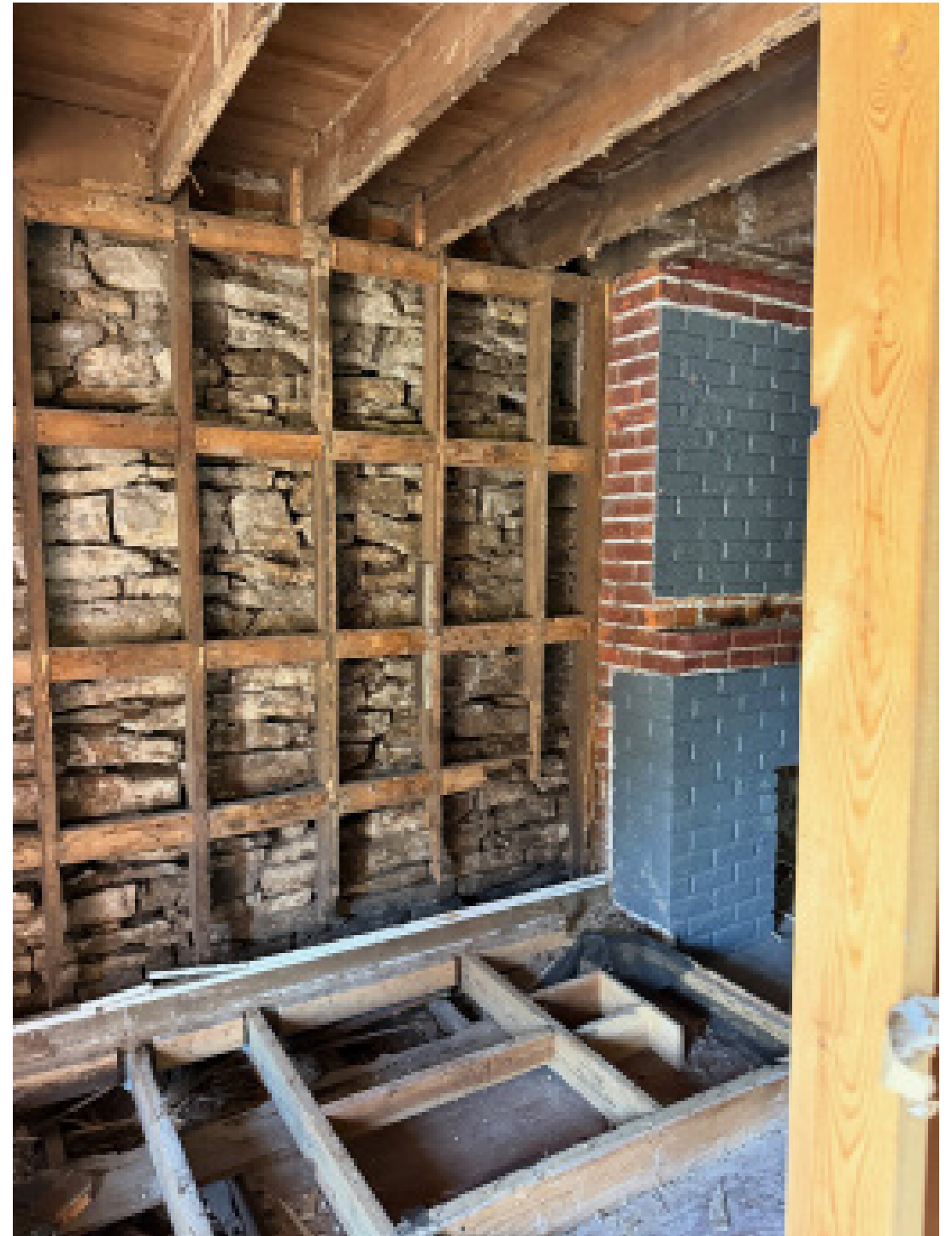
There is no easy way to add drainage or water proofing to the stone without excavating from behind, which will destabilize the wall and the wood frame structure above it.
