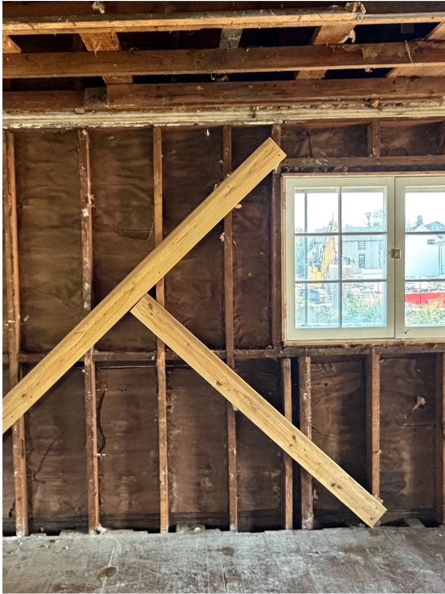
Lack of sheathing behind siding would not meet structural requirement for new use.
