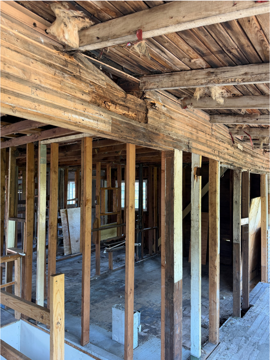
Header wall/ beam and rafters are severely rotten and sagged.
