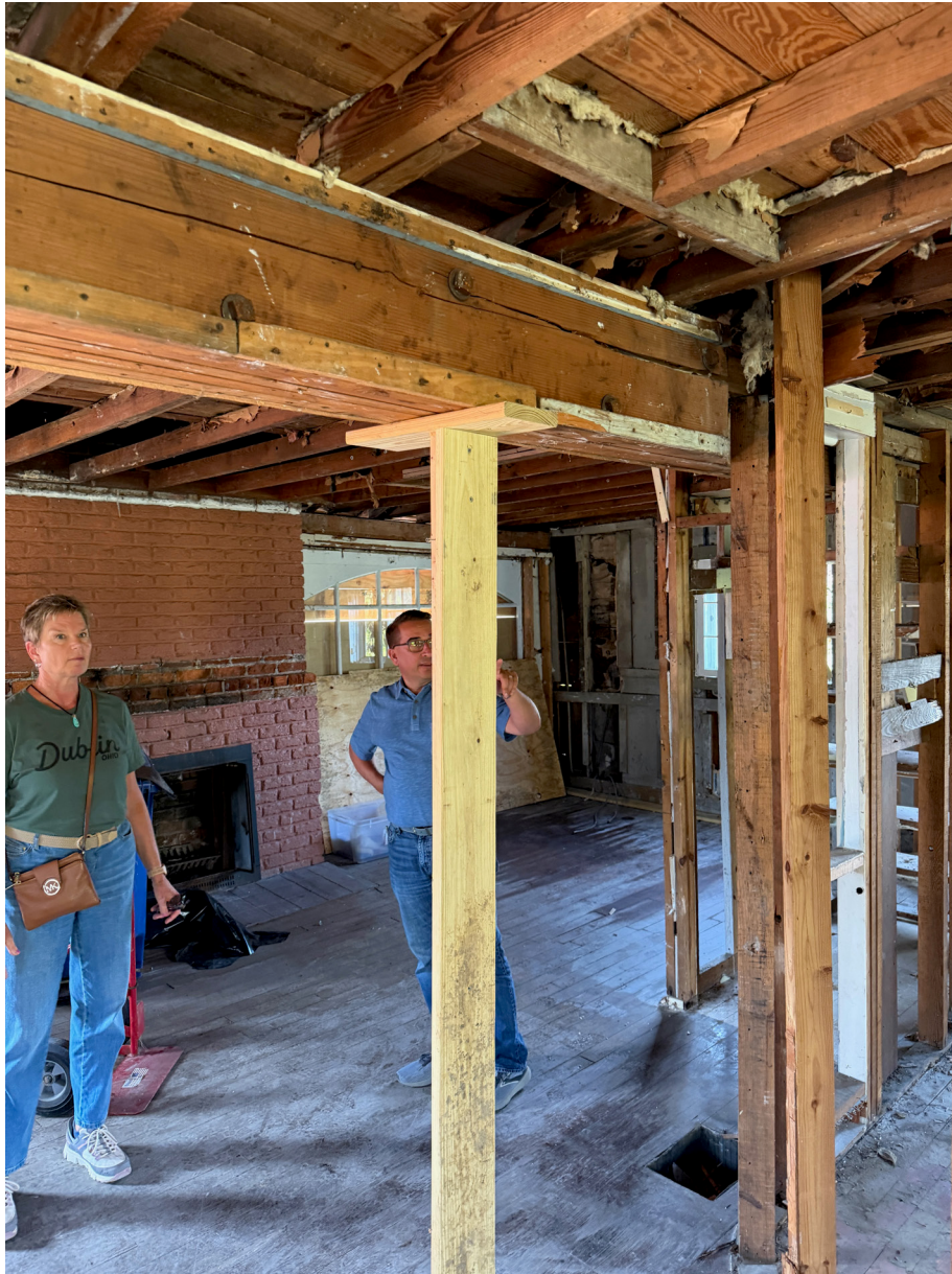
The giant wood beam supporting ceiling joists are not supported by anything but nailed into the wood stud.
