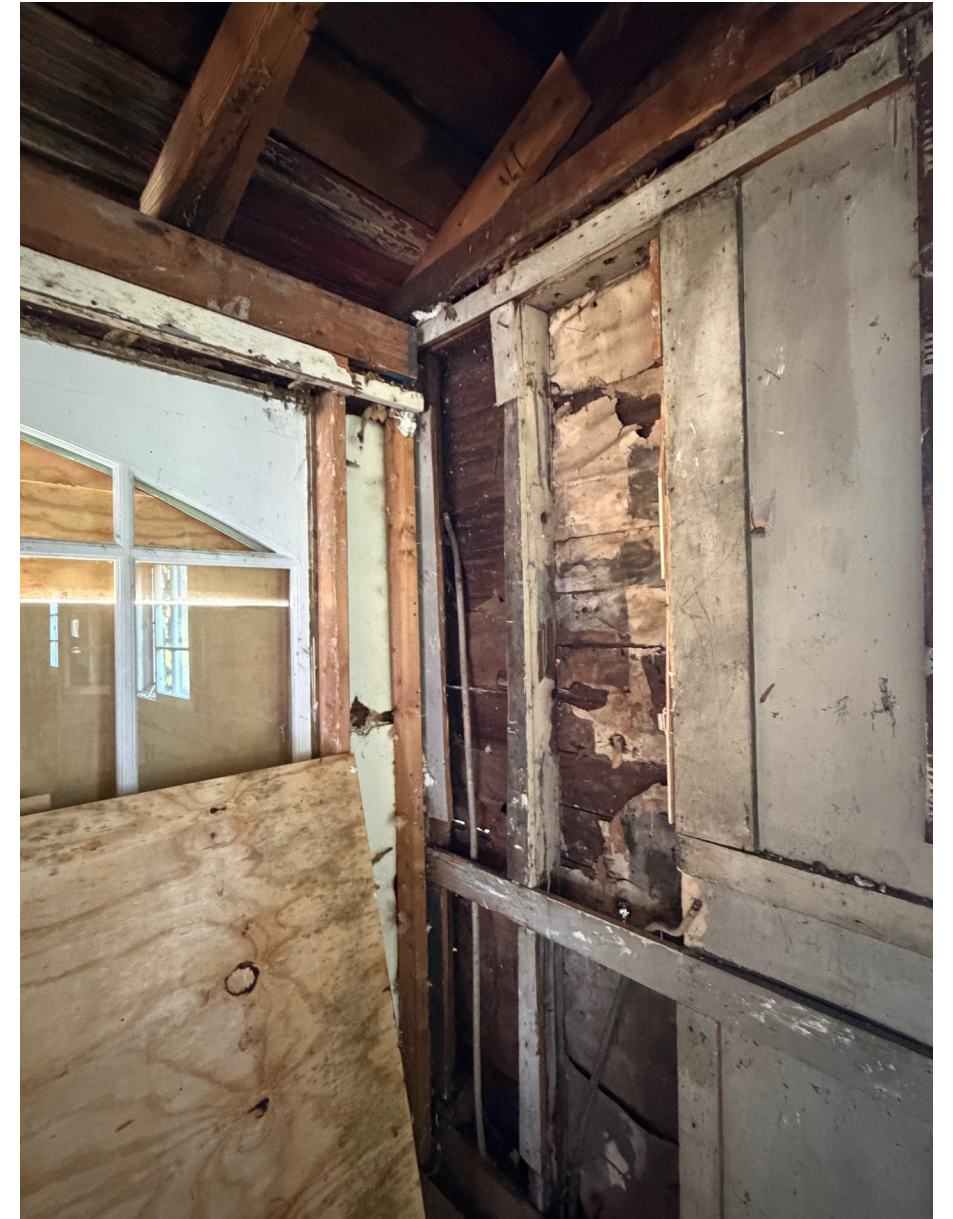
Framing inside some walls are cobbled together and would required complete replacemenn.
