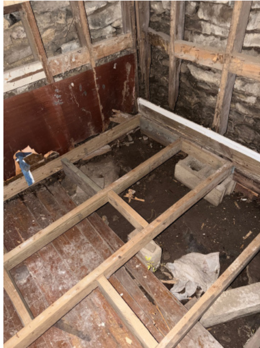
Floor joists are without proper support. Crawl space below shows deposit of soil and shattered rock.
