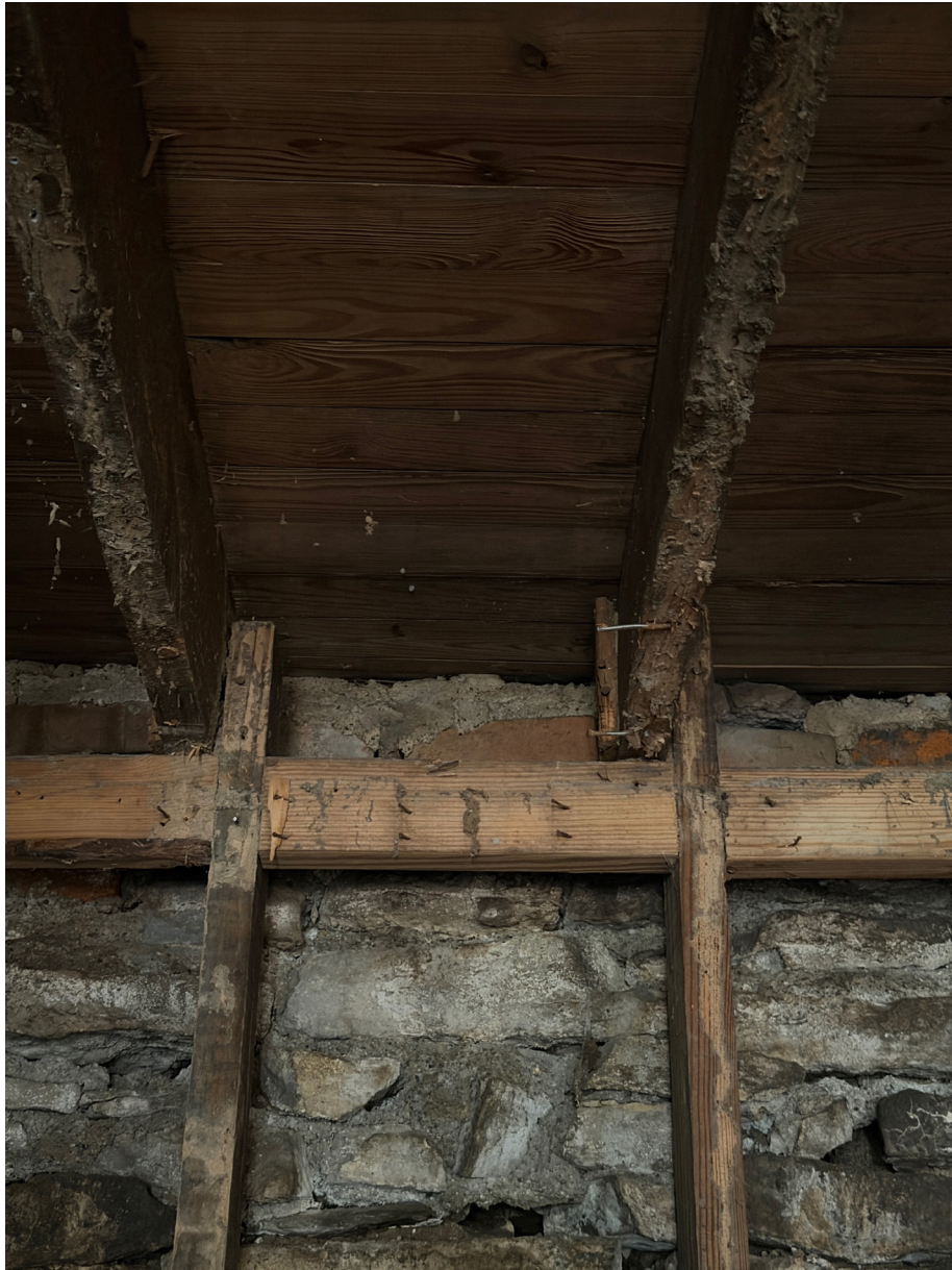
Wall framing is hung from the floor joist above, while the bottom all rotten away and nothing to bear on.
