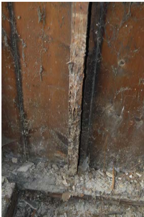
Photo 2- Insect damage on some structural studs, there appears to be no active insects at this time.
