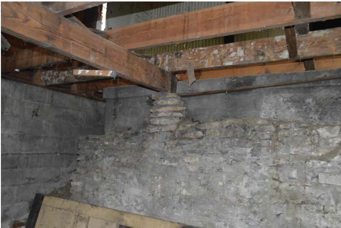
Photo 4- Basement foundation will require some repairs
