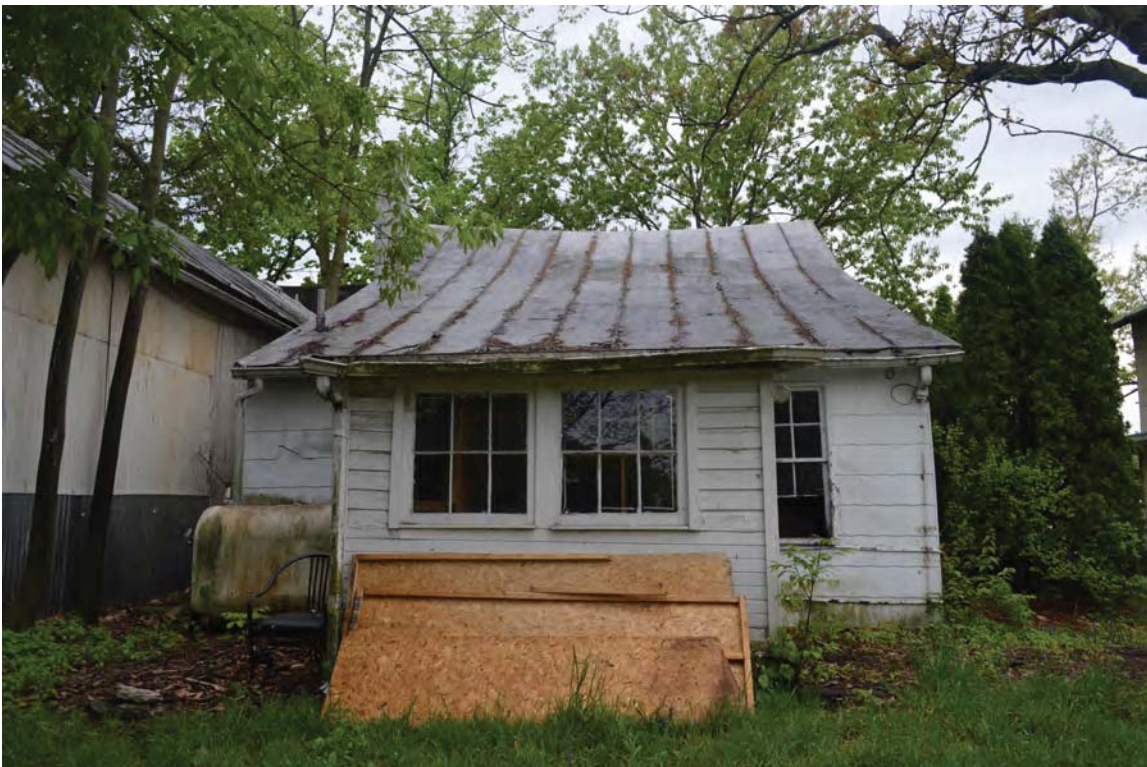
Photo 6- Rear of the 32 S High Building, note the later addition that hides the central cabin.
