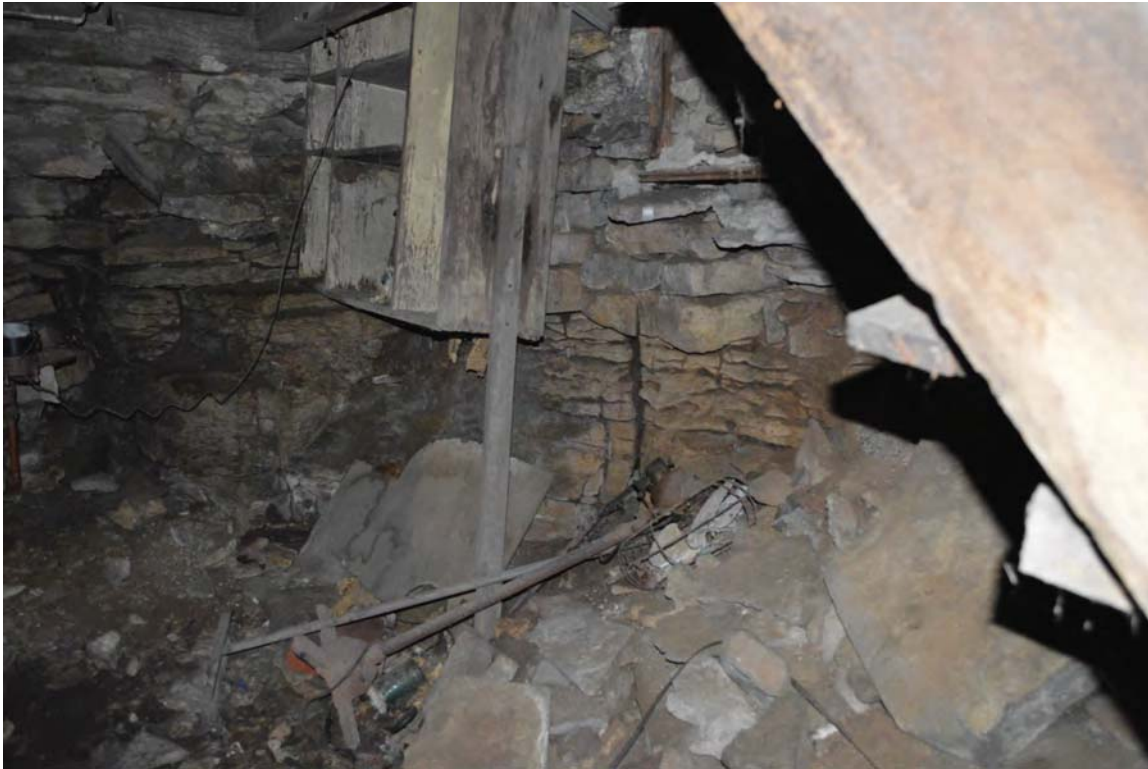
Photo 3- Additional photo of foundation damage
