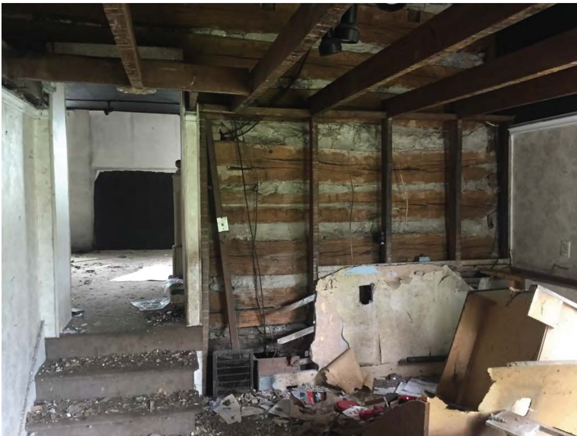
Photo 4- Exposed cabin logs, will require rethinking.
