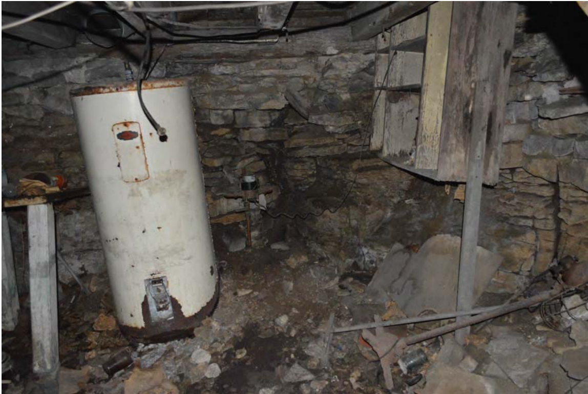
Photo 1- Foundation wall has fallen away at the base
