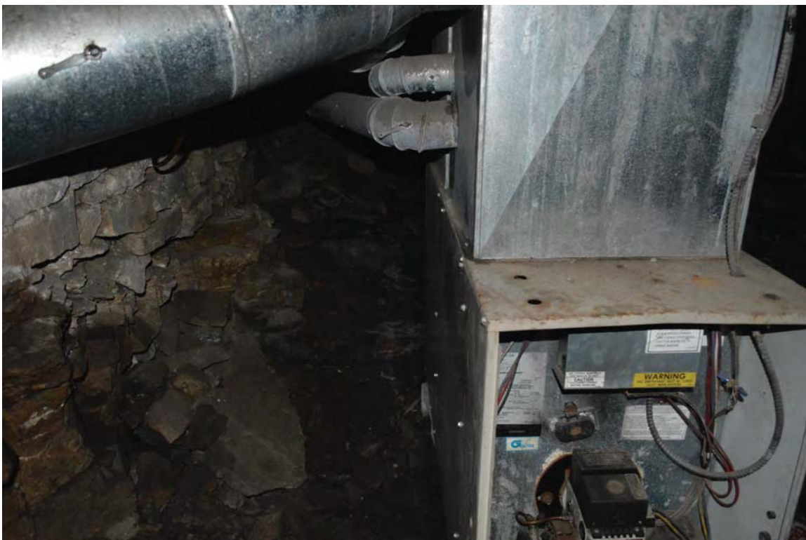
Photo 2- Additional foundation stones falling away
