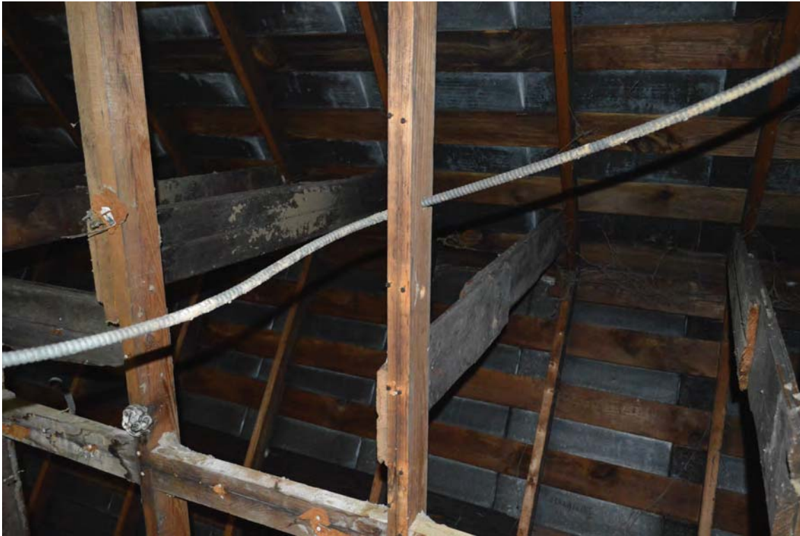
Photo 3- Existing roof framing will require some reframing and alterations to meet or exceed modern building code.
