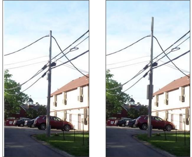
Figure 5.1B--Illustrative Type 1 Collocation Request on Existing Private Wooden Utility Pole (at right)
