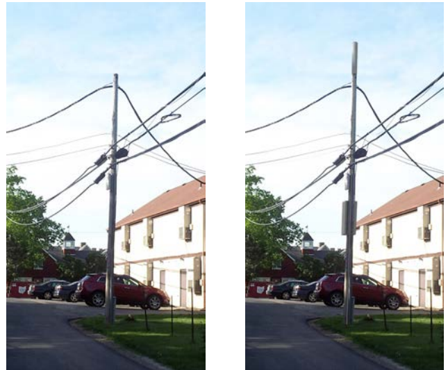
Figure 5.1B--Illustrative Type 1 Collocation Request on Existing Private Wooden Utility Pole (at right)
