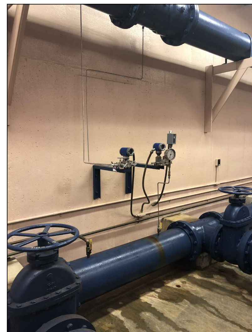
1 EXISTING DISCHARGE FLOW AND PRESSURE TRANSMITTERS
