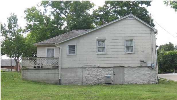
3. 106 S. High Street, east (rear) side. (Source: Jacobs Grant Design LTD, July 2019)
