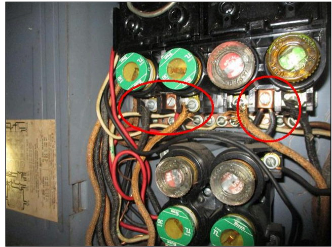
8.2 DISTRIBUTION PANEL Picture 2
