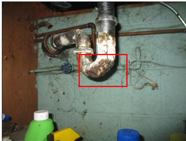
6.0 PLUMBING / SINK Picture 1
