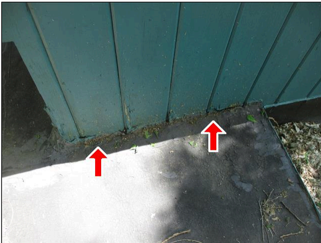
1.1 EXPOSED FLASHING Picture 1
