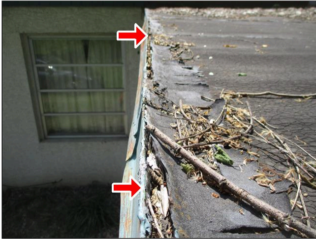
1.1 EXPOSED FLASHING Picture 3
