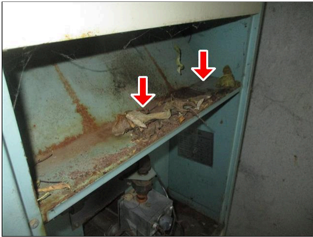
9.1.A BURNER Picture 1
