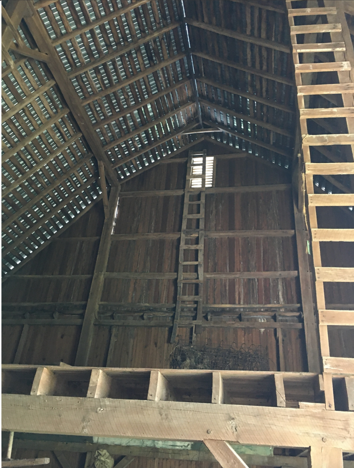
8. Interior view of barn, looking up into the loft. Note the circular marks on the heavy timbers from the saw mill as well as the mortise-and-tenon joints.
