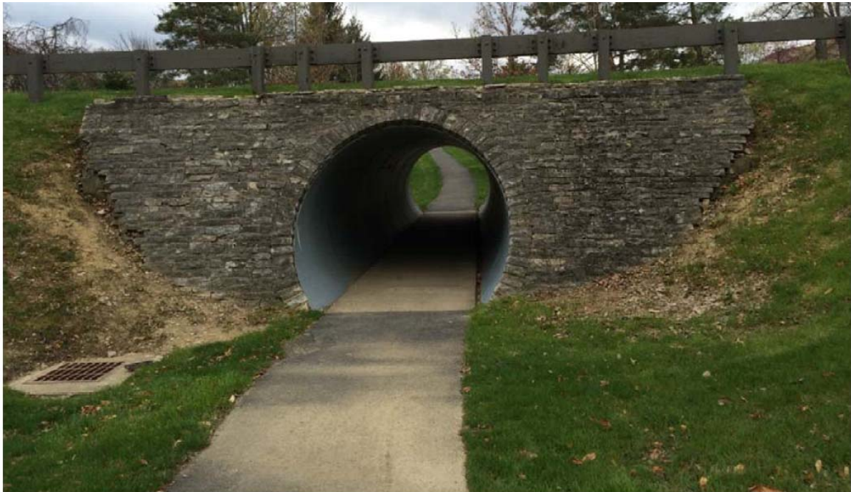
Typical headwall to be replaced and made vertical
