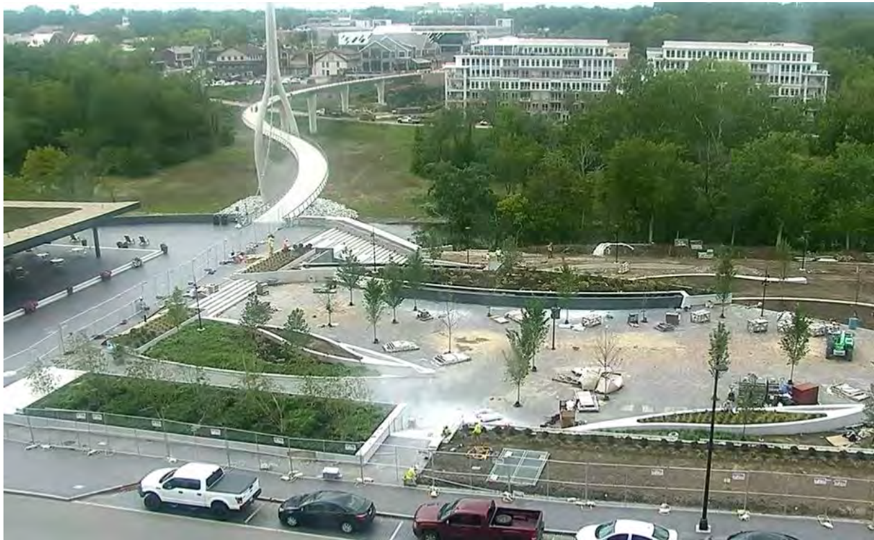
Riverside Crossing Park (under construction – August 30, 2021) and the Scioto Pedestrian Bridge (Dublin Link) Click on the link to go to live camera from the project site. http://bridgestreet.dublinohiousa.gov/riverside-park/
