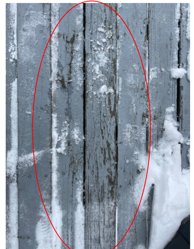
Many boards are rotting
