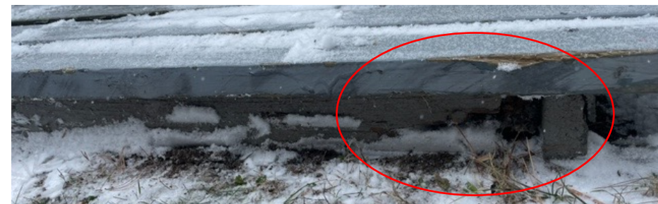
Wood support rotting
