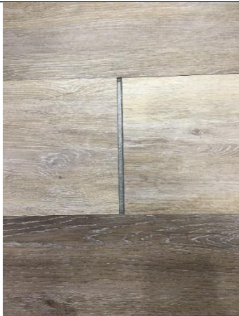
Photo 1 – Flooring planks separate about 1/4"
