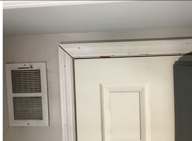
Photo 4 – Door frame joint separation about 1/4"
