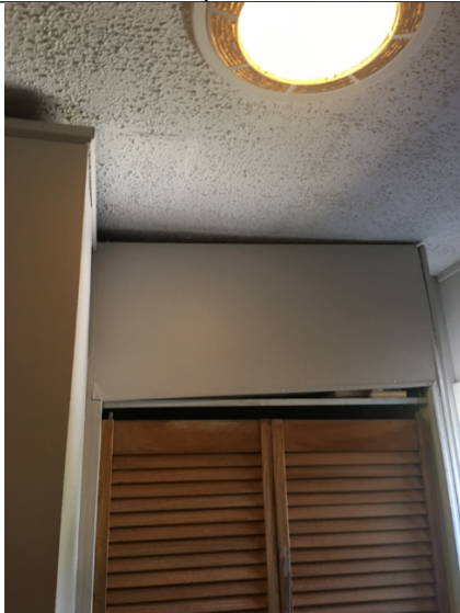
Photo 5 – Partition separation about 1"
