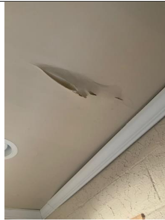
Photo 2 – Ceiling separation about 1/2"
