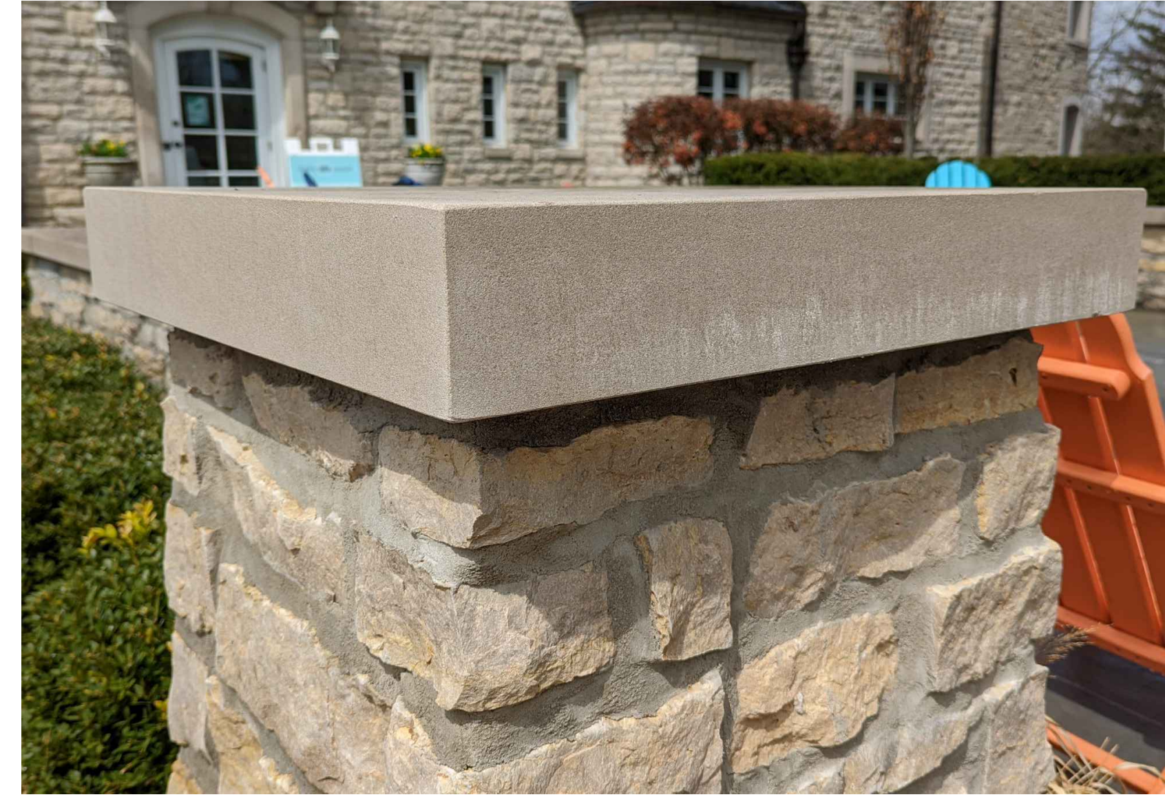
WING WALL CAP STONE TO MATCH EXISTING CAP STONE AS FOUND ON SITE. STONE SHALL BE BUFF LIMESTONE, SAWN ALL FACES. BASIS OF DESIGN LANG STONE INDIANA BUFF
