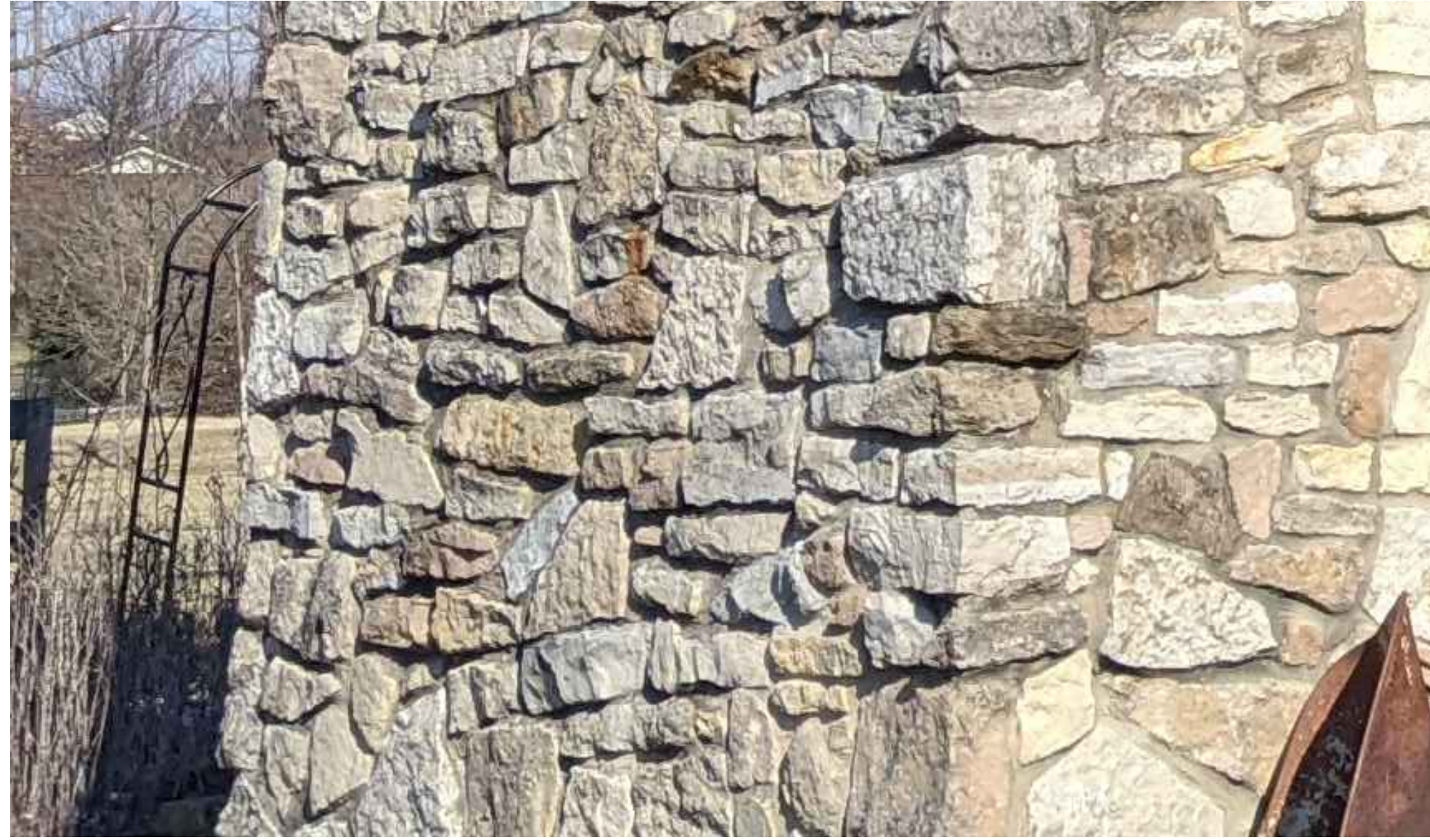
WING WALL AT CABIN LOWER LEVEL ENTRY TO MATCH STYLE AND PATTERN OF CABIN STONE. SEE ARCHITECTURAL PLANS.
