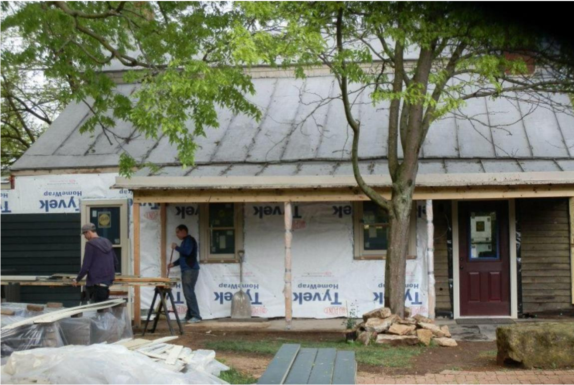
2. Construction photo of West Elevation, showing the rear porch, taken some time between 2012 and 2013. (Photo downloaded from Movoto website, accessed October 28, 2022, at https://www.movoto.com/dublin-oh/83-s-high-st-dublin-oh43017/pid_o41bdc5skh/#propertyPop )
